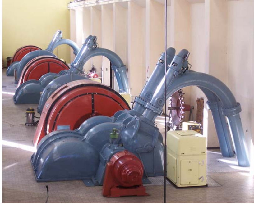
Figure 4: Pelton units of Mottec power plant.
